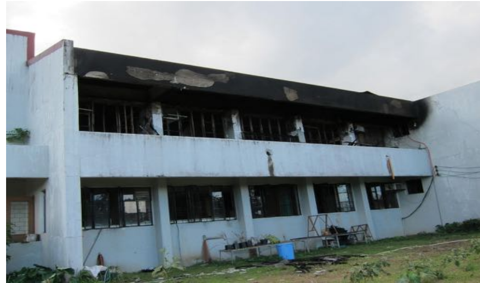
Fire at the Phillippine National Genebank in Los Banos (January 2012)
